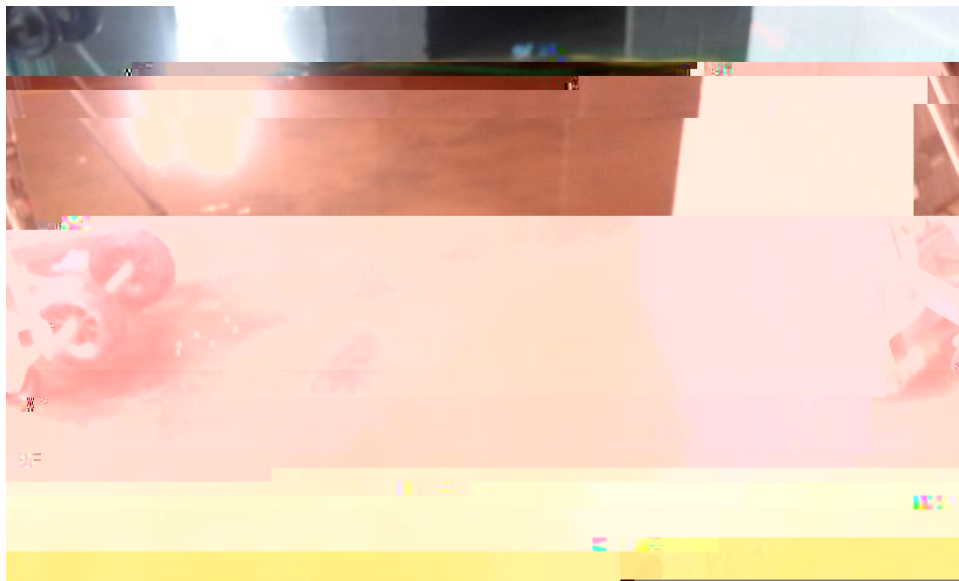
Corridor standing water (Typical)
