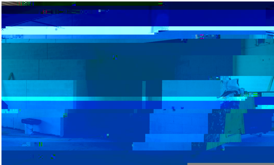
View of Area C below and above stairwell common areas as block fill is continued Also see drywall finished at corridor ready for paint.
